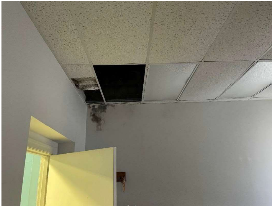
Photo 13 – View of suspected mold and water damage ceiling in Room 12.
