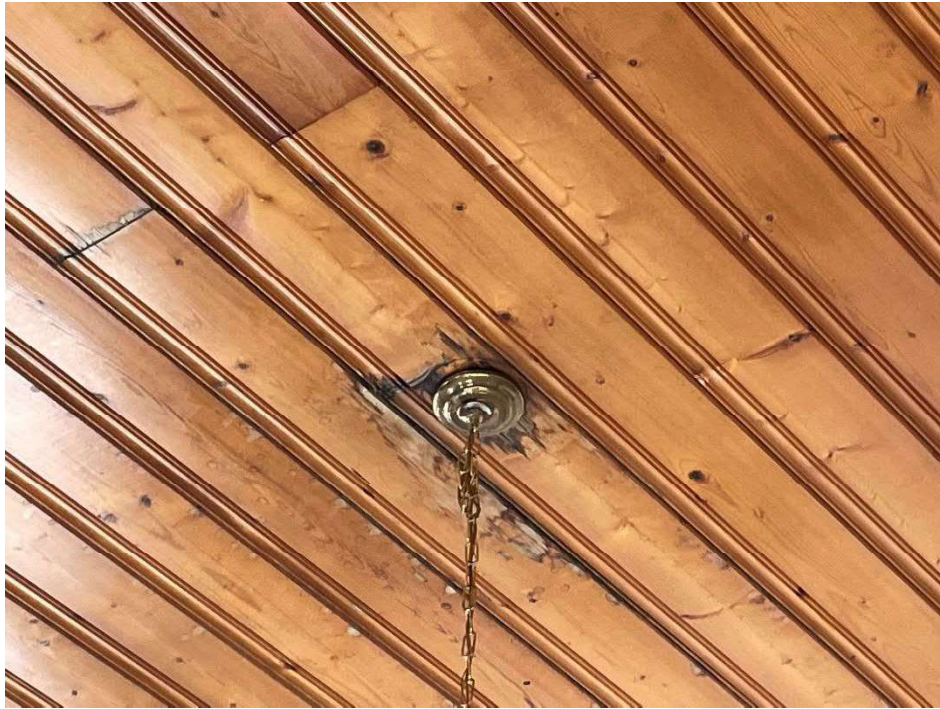
Photo 21 – View of water damage to the wood ceiling on the second floor landing. This ceiling is present throughout the first floor original section.
