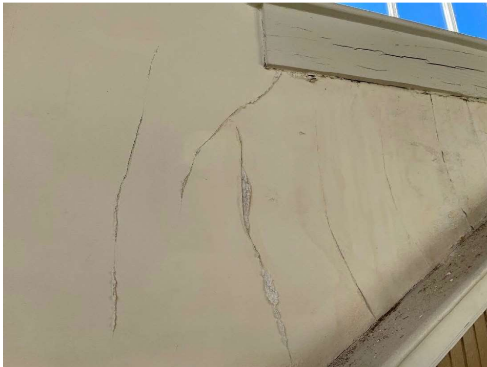
Photo 26 – View of plaster damage on the second floor landing.
