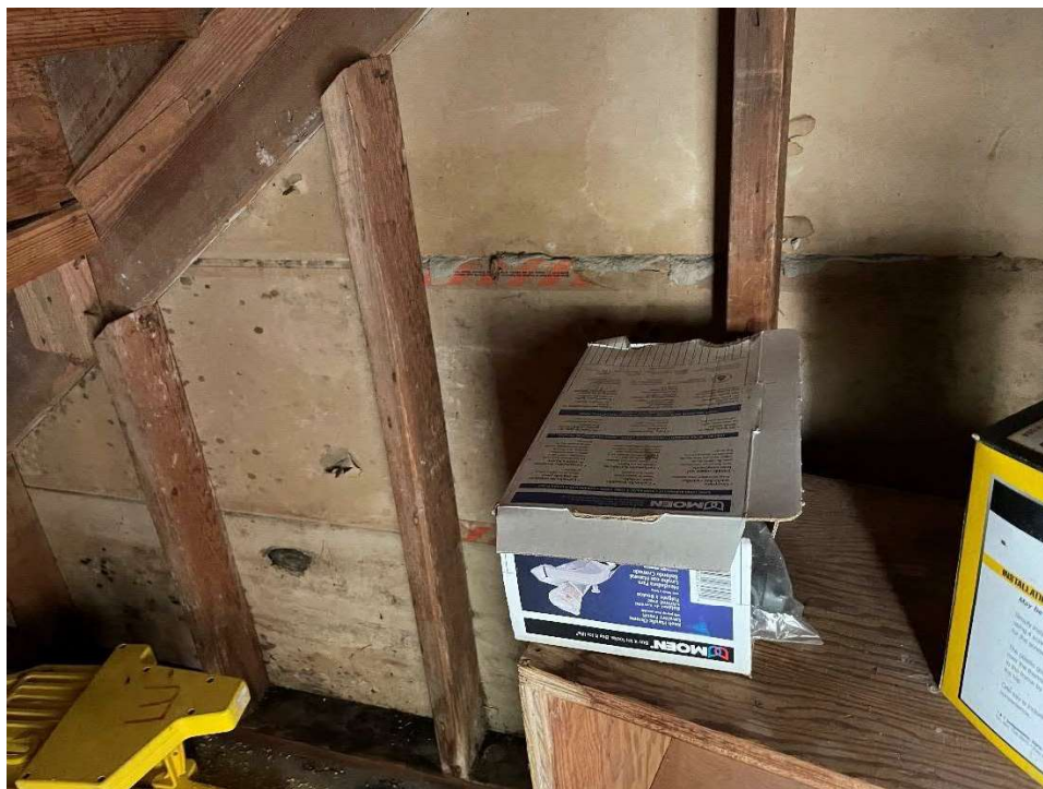
Photo 16 – View of the understairs closet by the bathroom with suspected mold growth on the gypsum lath.
