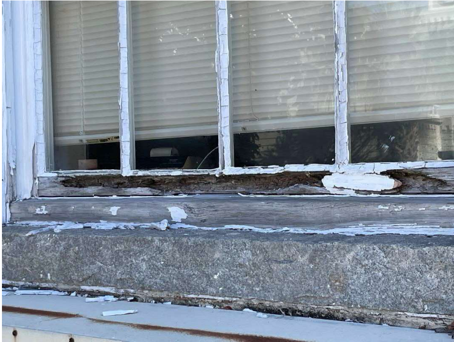
Photograph 3 – View of typical exterior window damage on the east side of the building of the original section.
