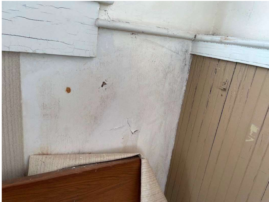
Photo 25 – View of plaster on the second floor landing behind the wallpaper.
