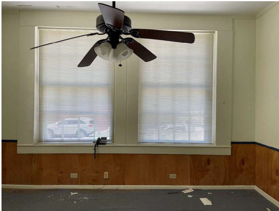
Photograph 6 – View of typical humidity impacted ceiling fan in Rooms 1 and 2.
