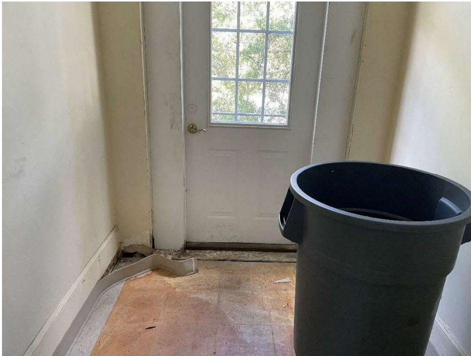
Photo 31 – View of the second floor back door with evidence of water damage around the base.
