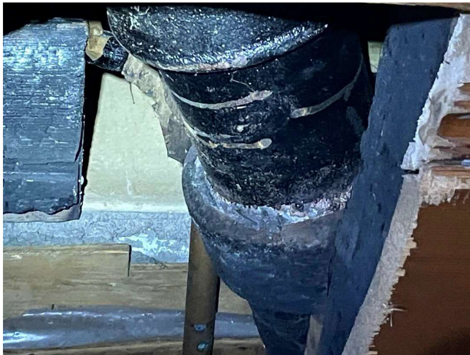
Photo 18 – View of the suspect ACM pipe insulation (black wrap) within the interstitial space between the first and second floor, above the wooden ceiling.
