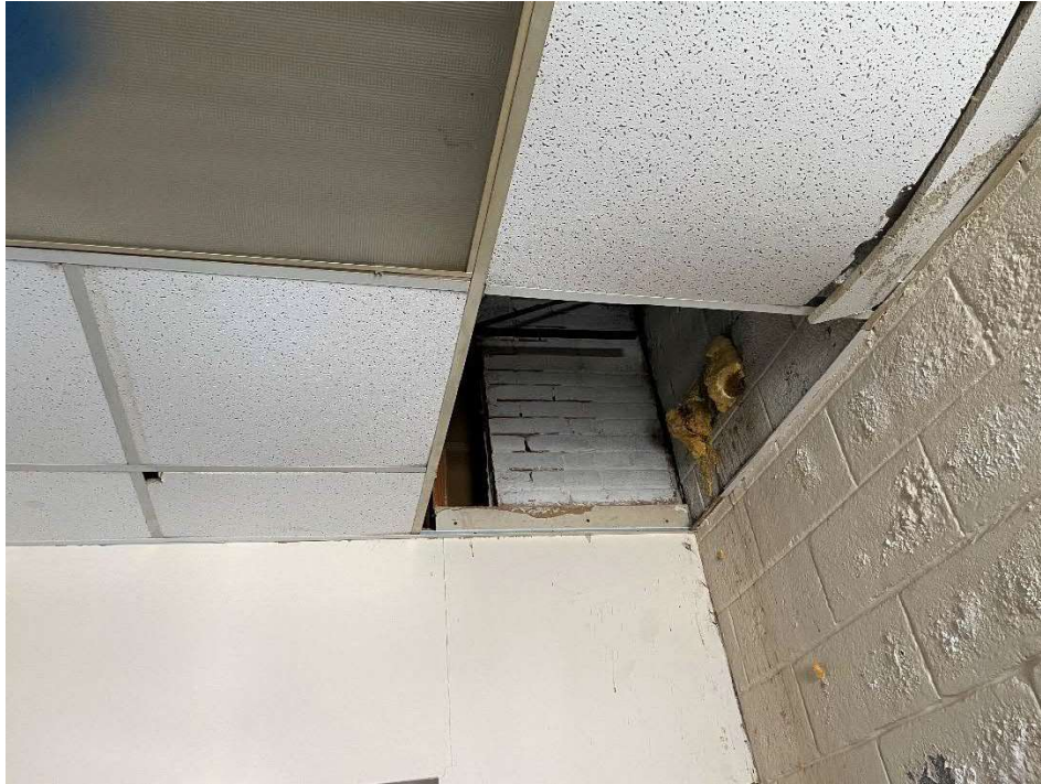
Photo 33 – View of the second floor back area joint of original building to east wing addition, area of suspected mold growth on the first floor.
