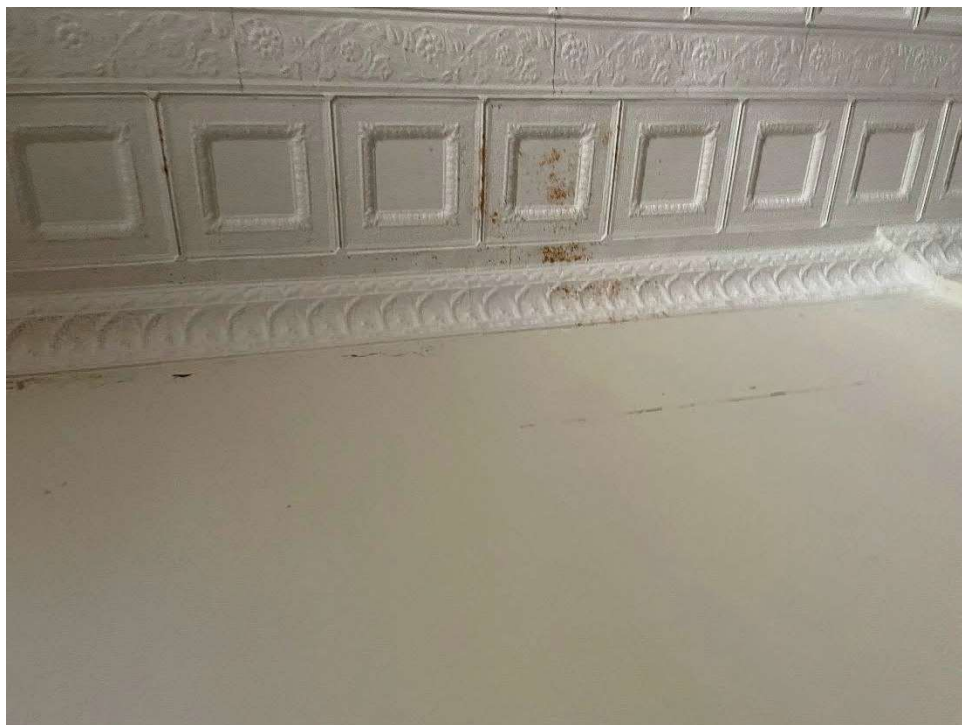
Photo 28 – View of rust on the ceiling tiles in the courtroom.
