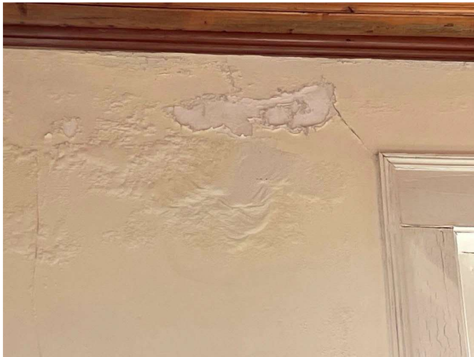
Photo 24 – View of water damaged plaster on the second floor landing.
