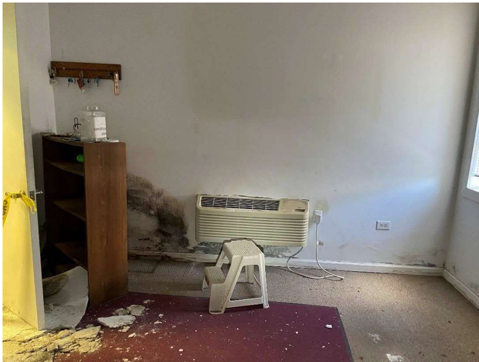
Photo 12 – View of the suspected mold and water intrusion in Room 12.
