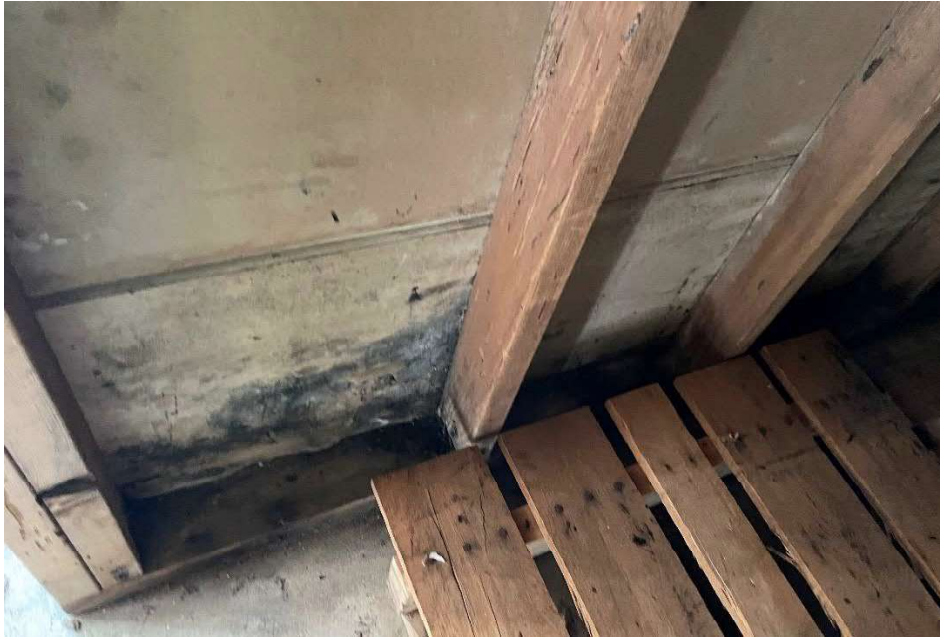
Photo 17 – View of the understairs closet by the bathroom with suspected mold growth on the gypsum lath.
