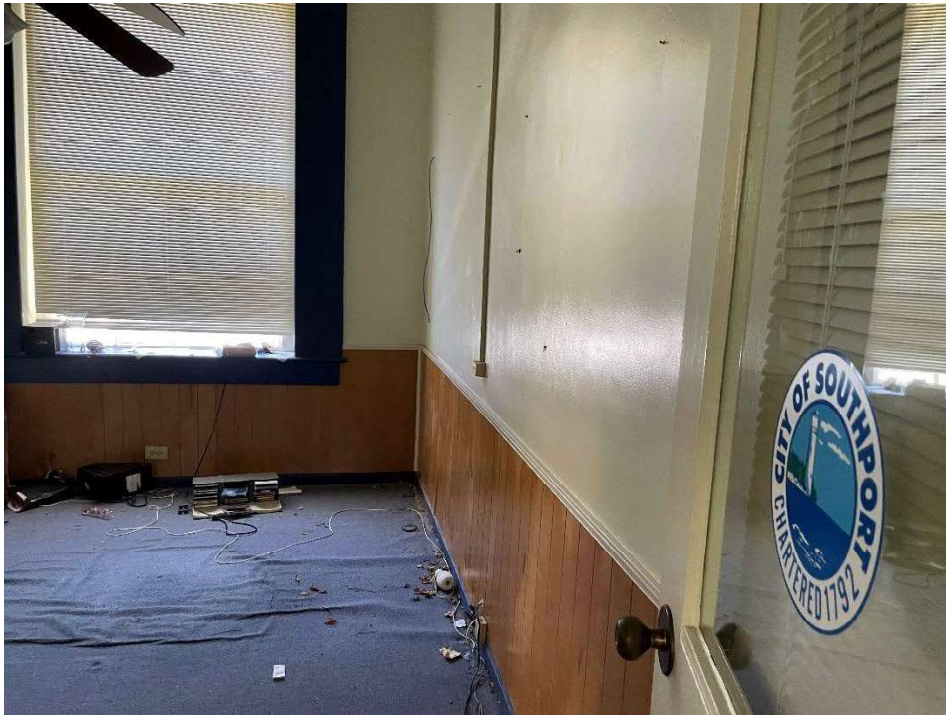
Photograph 5 – View of typical water damage in Rooms 1 and 2.
