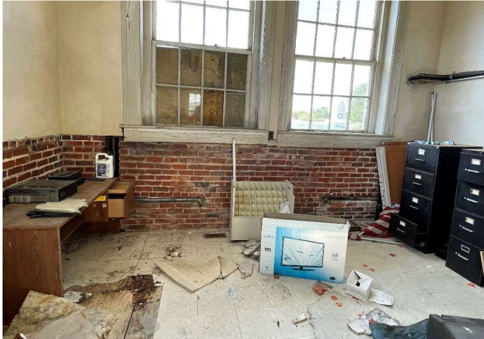
Photo 23 – View of significant water damage in the mechanical room on the second floor.
