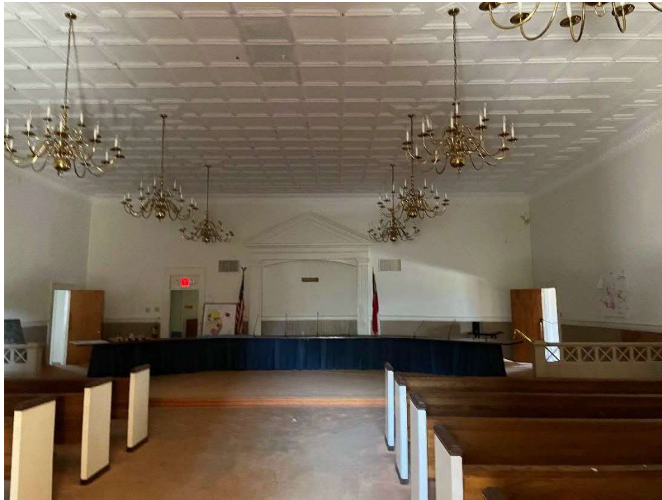
Photo 27 – View of courtroom on the second floor. Assume porous materials are mold impacted (carpet, fabric, benches, etc.).
