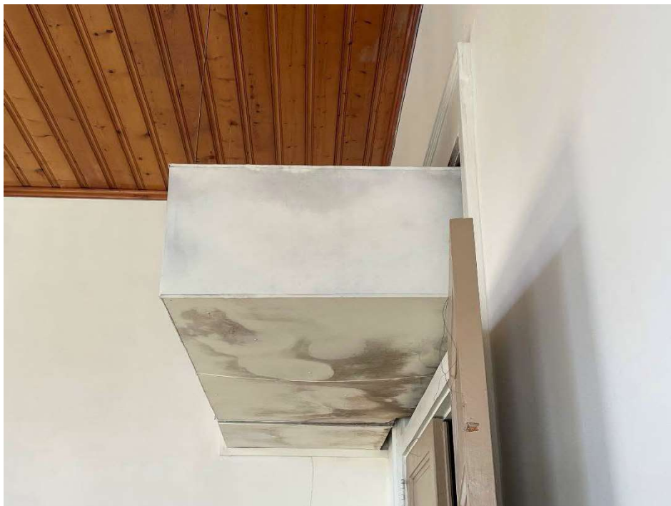
Photo 22 – View of suspected mold on the duct insulation leading into the courtroom.
