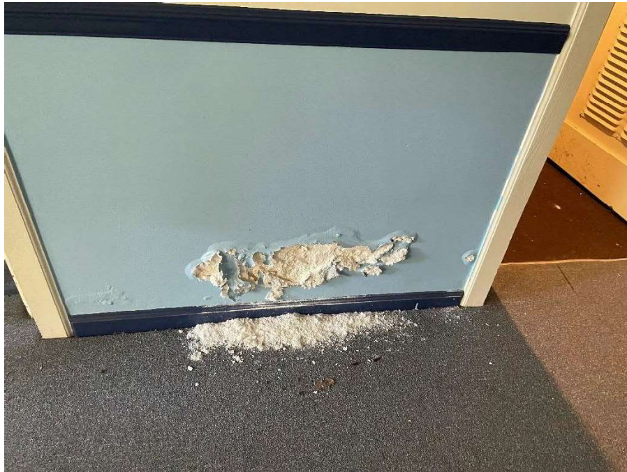
Photo 9 – View of water damage on wall in the first floor hallway.
