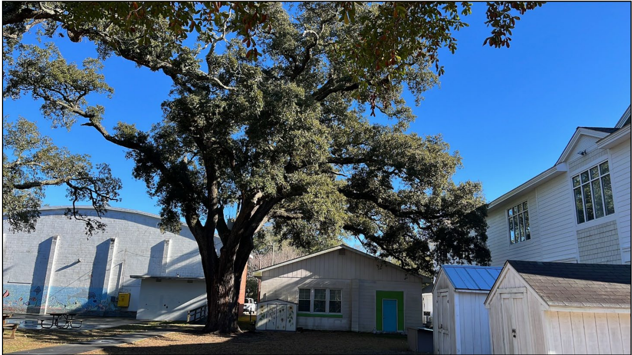
Photo 14: Looking northeast at live oak #35 showing the uneven crown and proximity to the building.
