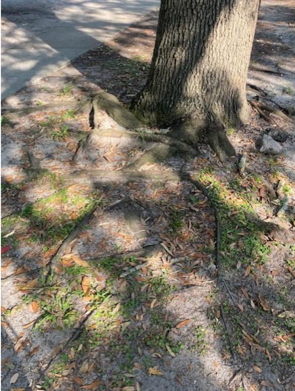
Tree 38: Exposed roots
