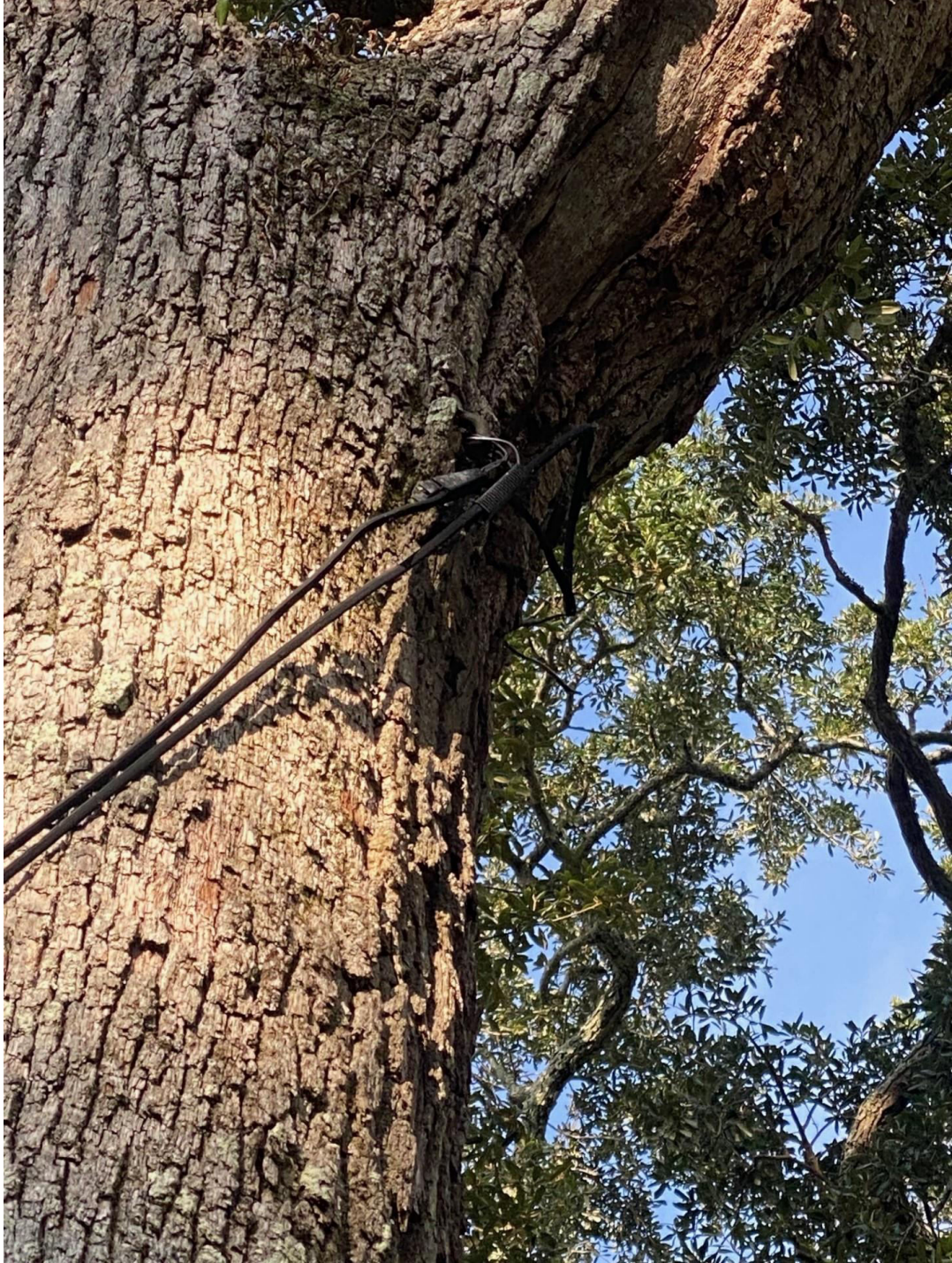
Tree 21: embedded wire/insulator. Bark loss.
