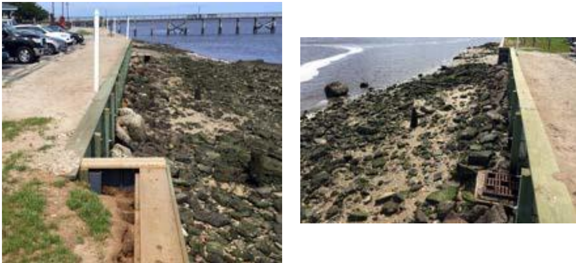
Figure 6: Photographs of the typical bulkhead sections (30 May 2018). Left – the transition between the vinyl section and wooden section with eroded upland fill. Right – typical rubble found at the foot of the structures along with the stormwater outfall.
