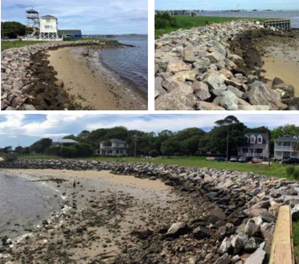
Figure 5: Photographs of the rock revetment protecting the wastewater pumping station (30 May 2018) Top Left – view facing east of the revetment and beach with the Wilmington Cape Fear Pilots Association in the background. Top Right – close-up view of the revetment and the transition to the vinyl wall. Bottom – view facing west from the vinyl wall of the revetment with pumping station in the background.
